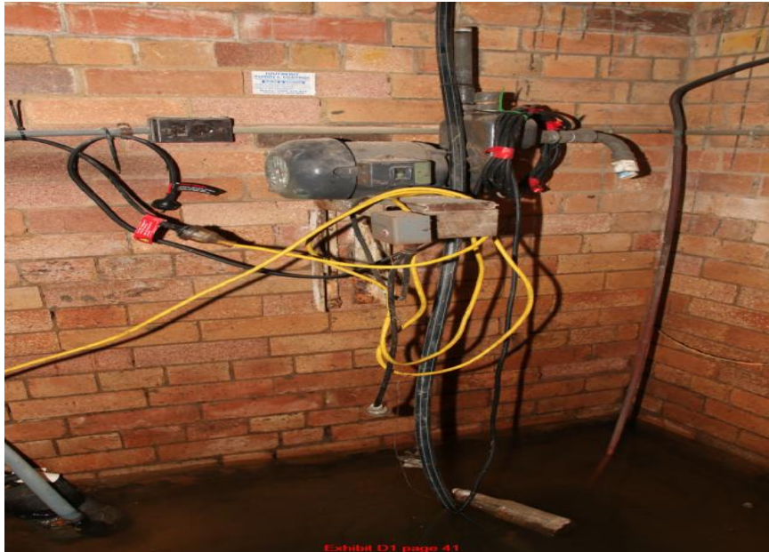
Yellow extension lead plugged into submersible pump
