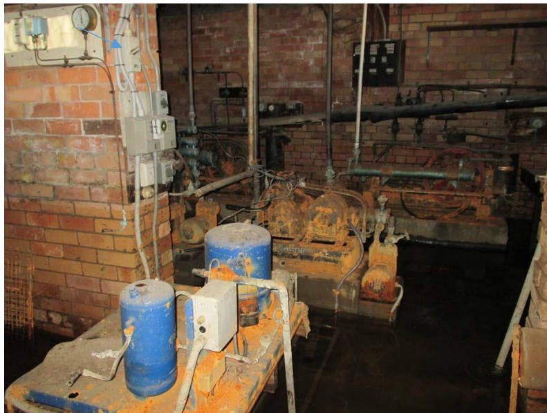
Isolator Switch to activate Blue Refrigeration unit
