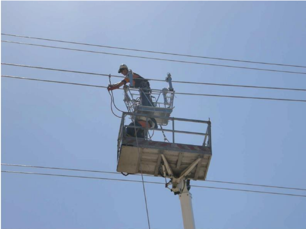
A closer image depicting Mr Cheney in the conductor cart and Mr Parungao in the Elevated Working Platform. Mr Cheney is unclamping and detaching the earthing lead from the conductor.
