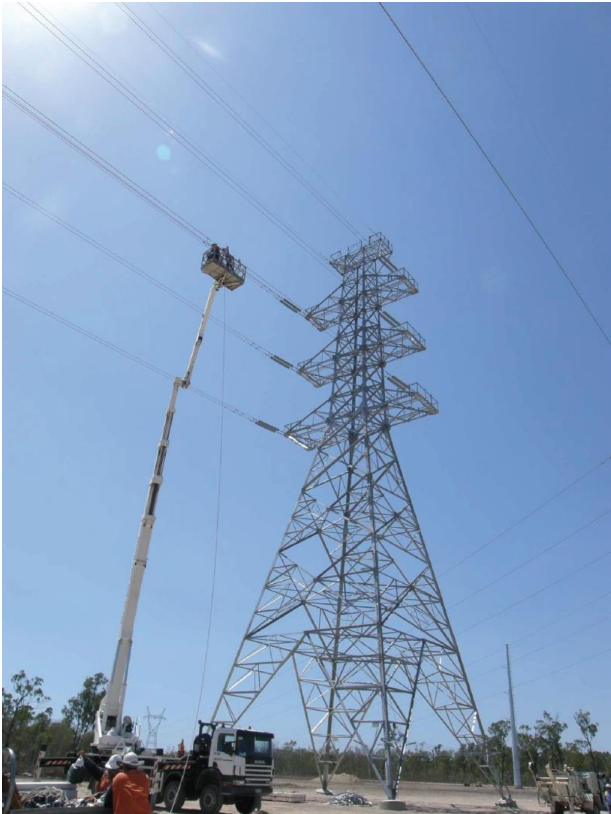
The scene showing the positioning of the Elevated Working Platform positioned under conductors moments before the incident
